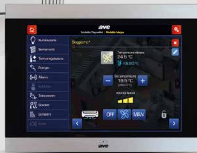
Supervisione mediante Touch Screen Supervision by Touch Screen
